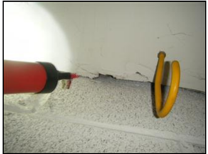
3.0 Picture 2 Air leakage along garage ceiling perimeter
