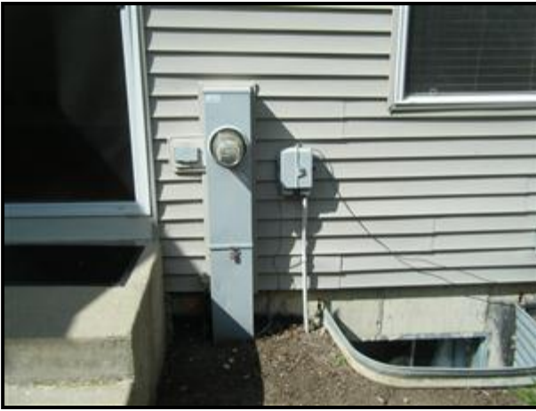
7.0 Picture 1 Service meter
