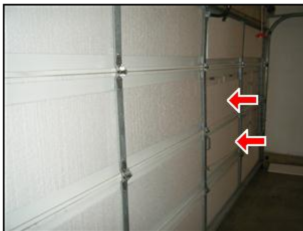
3.4 Picture 1 Delaminated foam board
