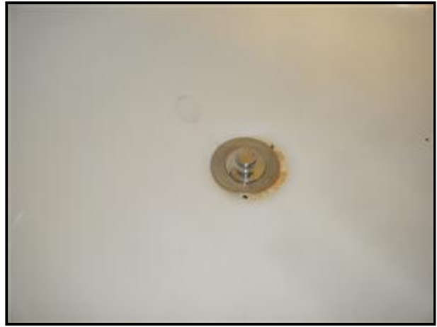
6.1 Picture 2 Light rust at tub drain
