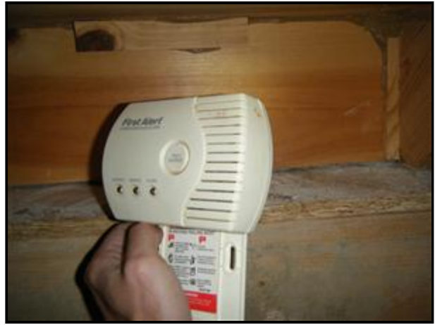
7.8 Picture 2 Battery CO detector in basement - w/o battery
