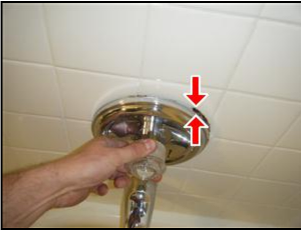
6.1 Picture 1 Loose faucet
