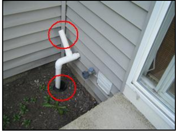
6.4 Picture 2 Air vents
