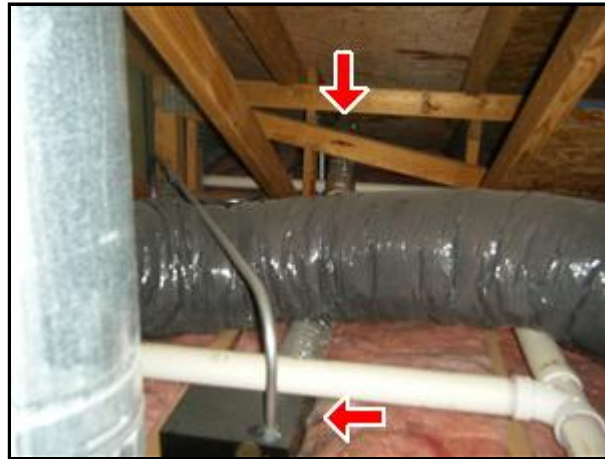
9.5 Picture 3 Master bath fan &amp; exhaust
