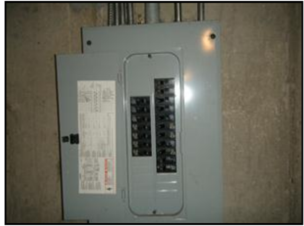
7.0 Picture 2 Main service panel
