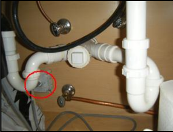
7.5 Picture 1 Disposal outlet
